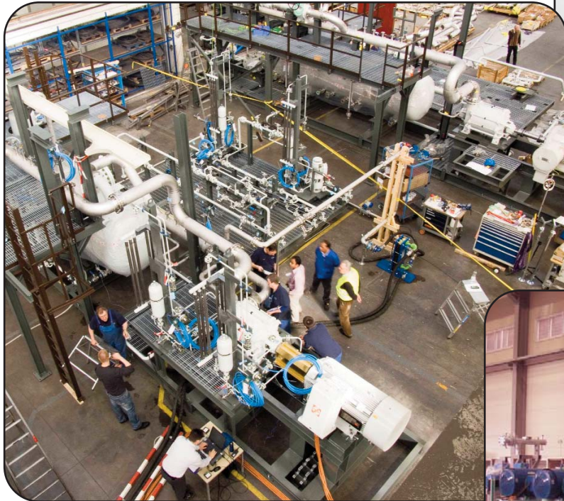
Compressor system for Vent Gas Recovery
